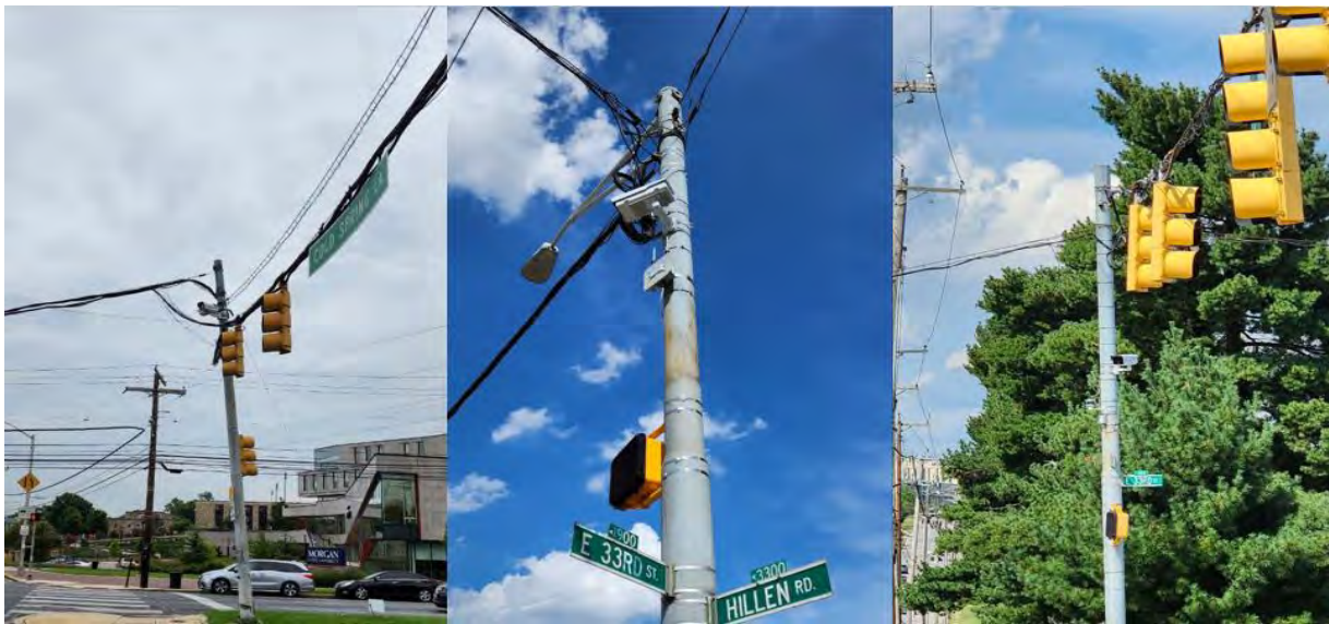
Figure 3 CCTV Cameras Installed at Both Intersections on the CAV Testbed
