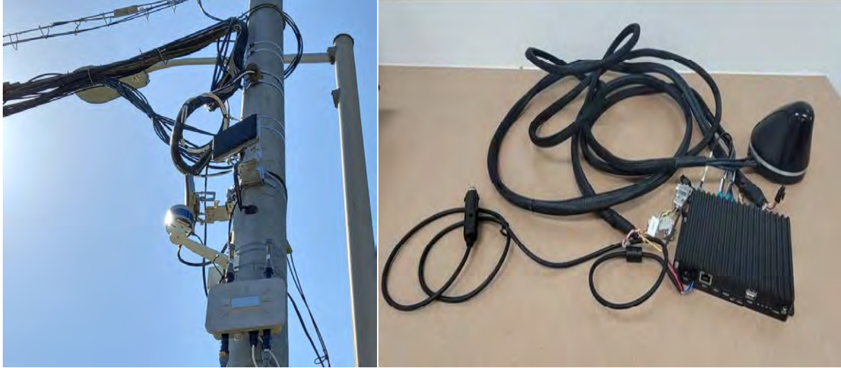
Figure 2 LiDAR Sensor, RSU, and OBU Setup on the Morgan State University CAV Testbed
